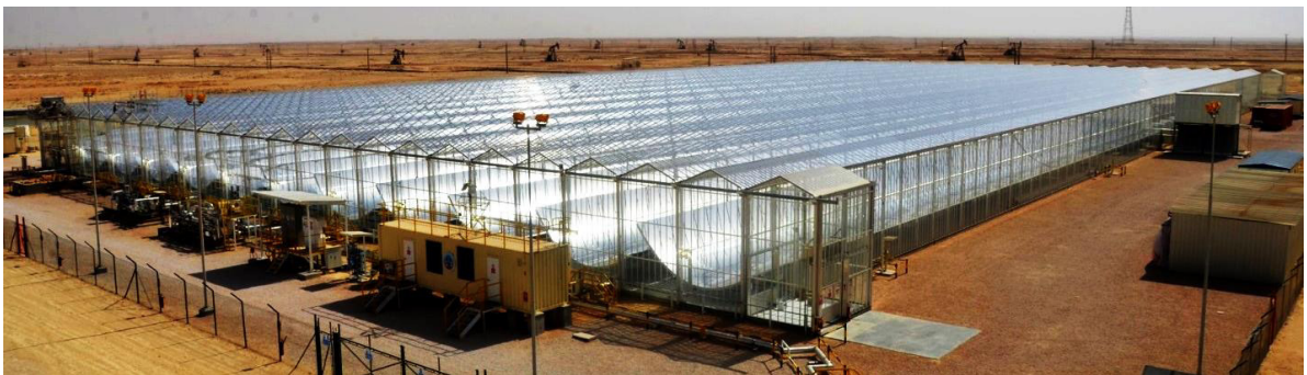
Figure 2: GlassPoint pilot plant, South Oman
